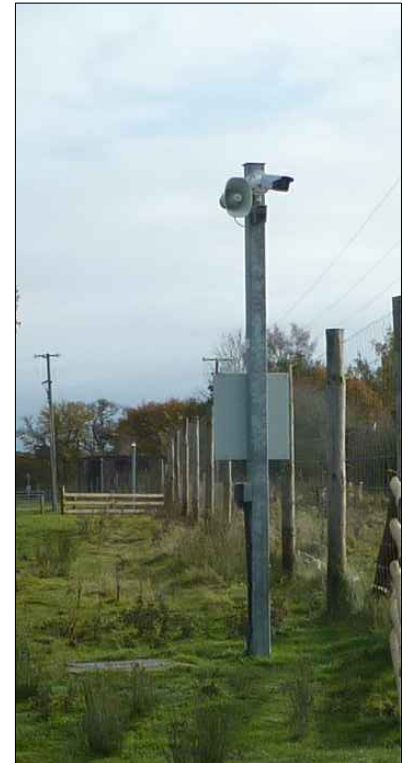
CCTV on adjacent site
