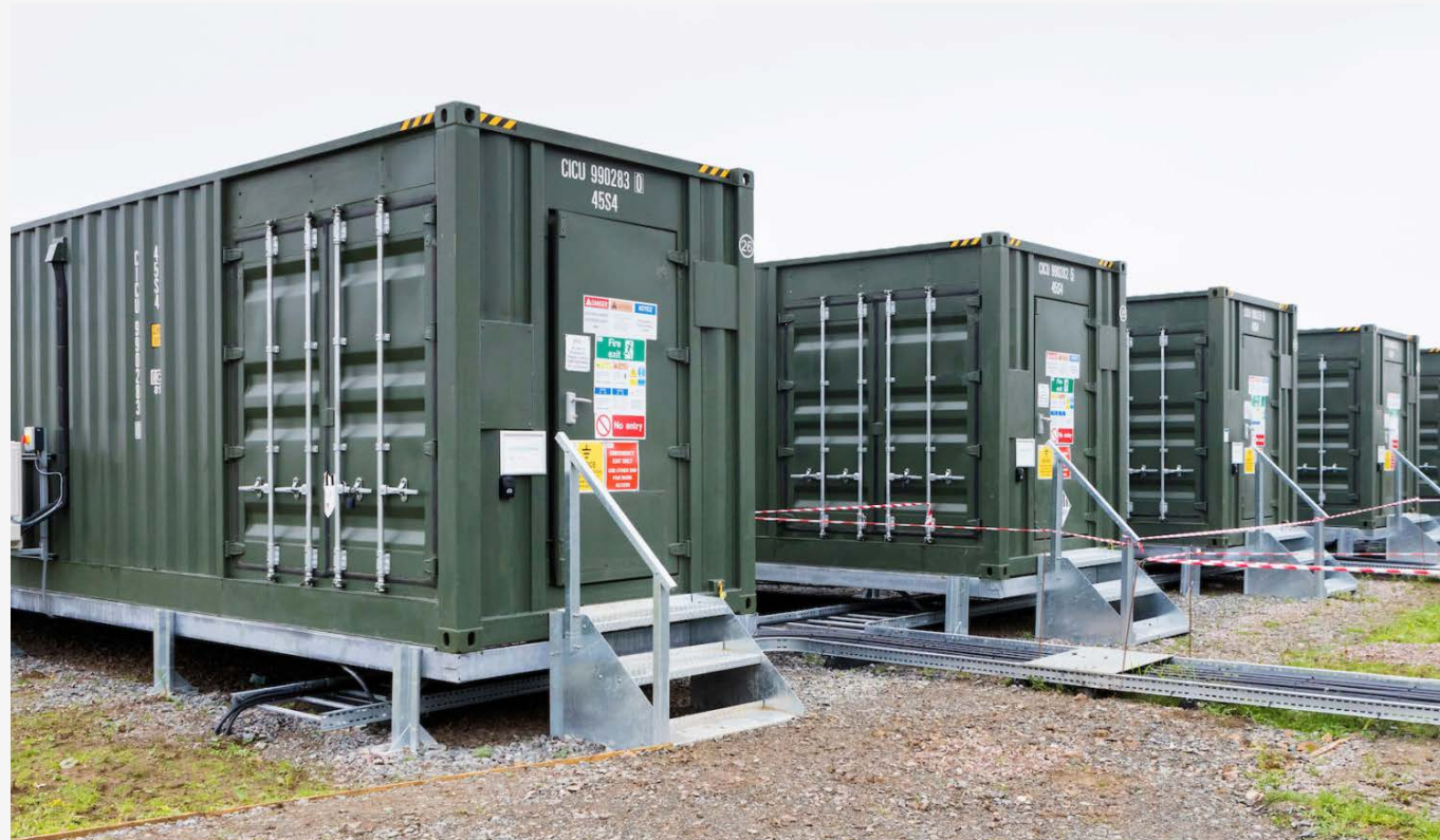
Figure 4: Example of a battery storage facility
